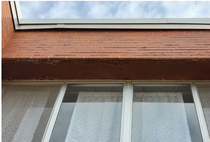
Fig. 13: Galvanic action occurring between the steel lintel and aluminum windows on the 1973 addition, which causes accelerated corrosion of both metals. Water intrusion into the brick above is also causing significant rust on the lintel and damage to the mortar.
