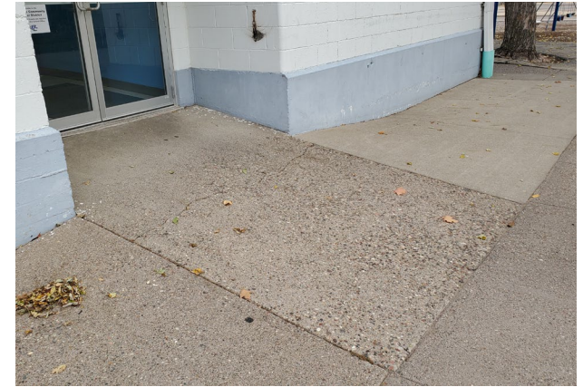
Fig. 4: The concrete pad outside of the south cafeteria door exceeds the maximum ramp slope allowed by code to act as an accessible means of egress.
