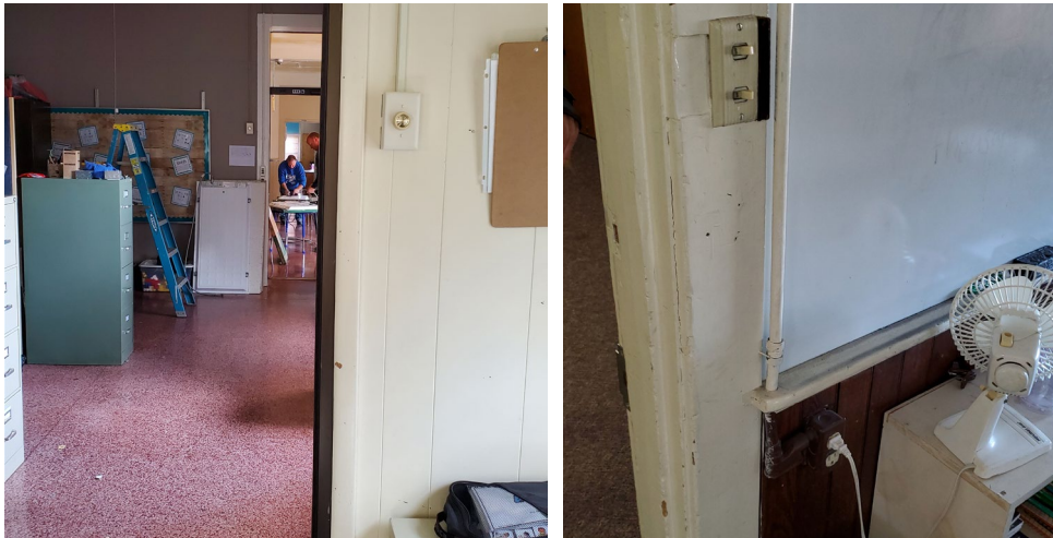
Fig. 24, 25: Wall devices such as light fixtures, fire alarm pulls, thermostats, fire extinguishers, and call buttons must be installed at a maximum of 48 inches off the floor to the operable portion of the device. These are two examples that exceed 48 inches and would need to be lowered.
