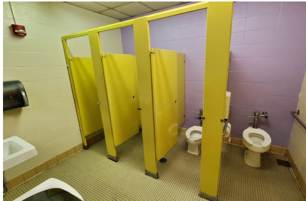
Fig. 17: A girls restroom adjacent to the 1960 classroom wing that does not have a wheelchair-accessible stall, adequate wheelchair turning radius, or compliant grab bars. Exposed piping under sinks must be covered with a protective shroud to prevent burns by wheelchair users.
