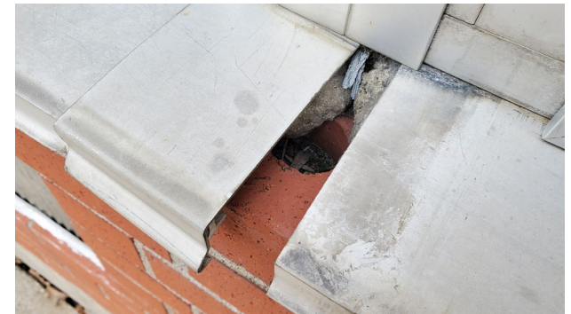
Fig. 9: Damaged window sill in 1960 addition, allowing water and pests into wall cavity
