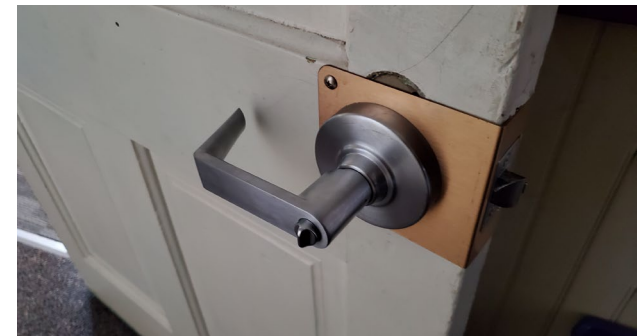
Fig 8: An existing door which has been modified with an ADA-compliant lever door handle.
