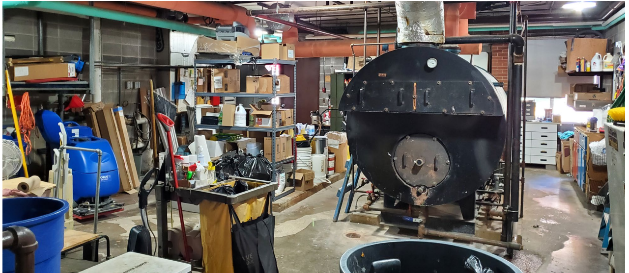
Boiler room in the 1973 addition.
