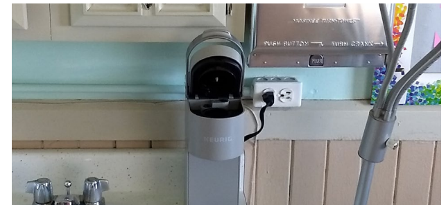
Non-GFCI outlet next to a lavatory.
