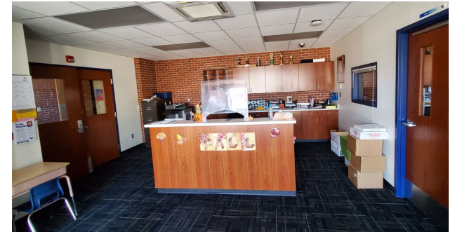
Fig. 20: The reception casework in the administration office does not have an ADA-accessible transaction counter.
