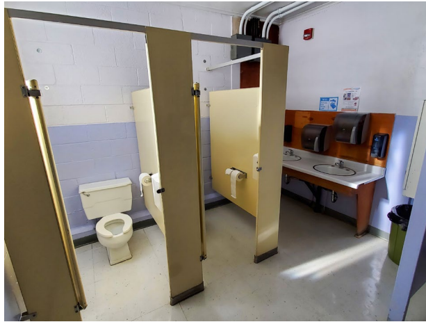
Fig. 12: A non-accessible women's restroom near the cafeteria. This restroom does not have a wheelchair-accessible stall with grab bars or adequate clear space at the sink fixtures.
