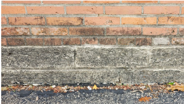
Left, Fig. 2: Mold and mildew growth at base of brick and limestone foundation.
