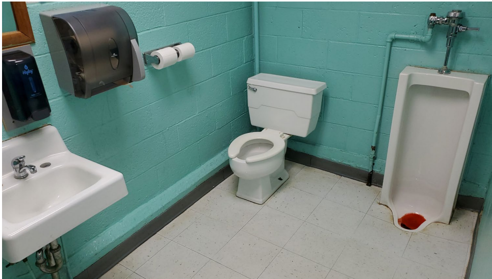
Fig. 23: This restroom has a number of issues that make it not compliant with ADA: 1) A toilet without the minimum required clearance away from the wall and clearance from the urinal. 2) No grab bars installed at the toilet. 3) Toilet paper dispenser installed higher than the maximum height. 4) Mirror installed higher than the maximum 48 inch height. 5) No protective shroud around the piping under the sink.
