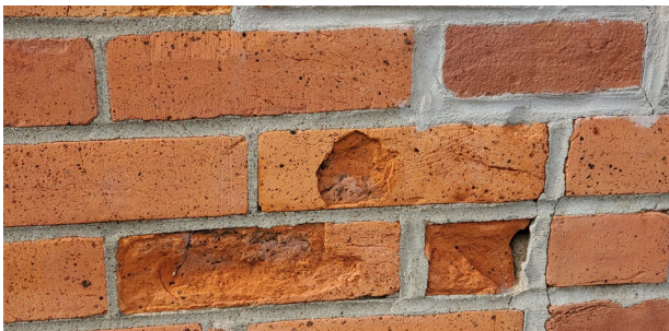
Fig. 4: Spalling brick on the 1848 exterior wall.
