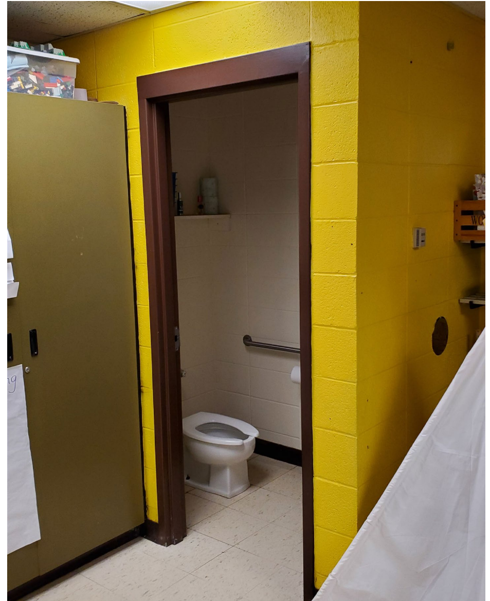
Fig. 18: A non-compliant single-use restroom in one of the 1973 classrooms
