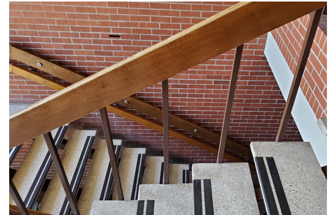
Fig. 2: The egress stairs in the 1973 addition have risers that are open to below and are not compliant with current codes. The vertical guardrail balusters are wider than code allows, and the handrails are a non-compliant shape and size for accessibility.
