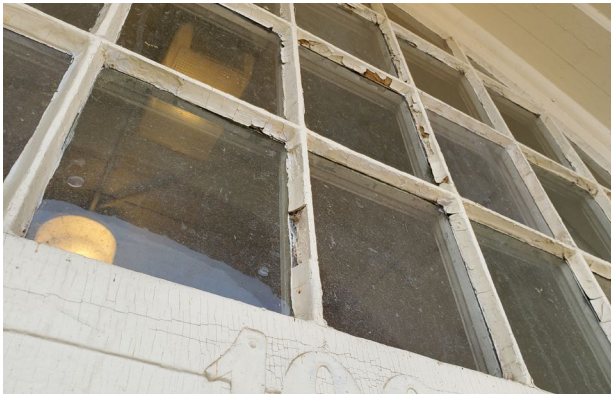
Fig. 3: Arched single-pane window on 1848 building with possible asbestos putty.
