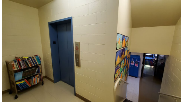
Fig. 1: The elevator and stair landing is not enclosed with fire-rated doors and does not have a two-way communication device for a disabled individual to call for help, which is required for non-sprinkled buildings.
