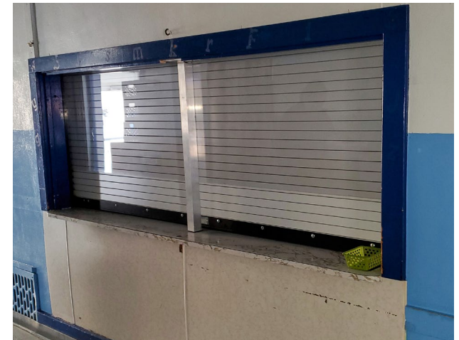
Fig. 13: Both the kitchen serving window and the dish return window have a counter height that is higher than the 34" maximum allowed by
