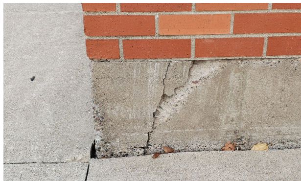
Fig. 7: Cracking and spalling concrete foundation on the 1960 addition
