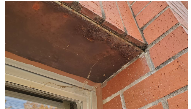
Fig. 10: Rusting steel lintel on the 1973 addition
