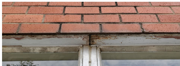
Fig. 8: Damage to window head lintels due to water intrusion into the brick cavity on the 1960 addition. Cracking window gaskets are also visible.
