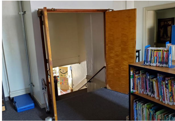
Fig. 3: Door opens wrong direction for fire egress and does not have compliant stair landings. Egress corridor space is being utilized as a library.
