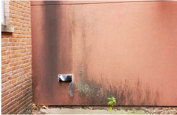
Fig. 12: Mold and mildew growth on the 2005 elevator addition EIFS panels due to a lack of gutters on the 1848 building.
