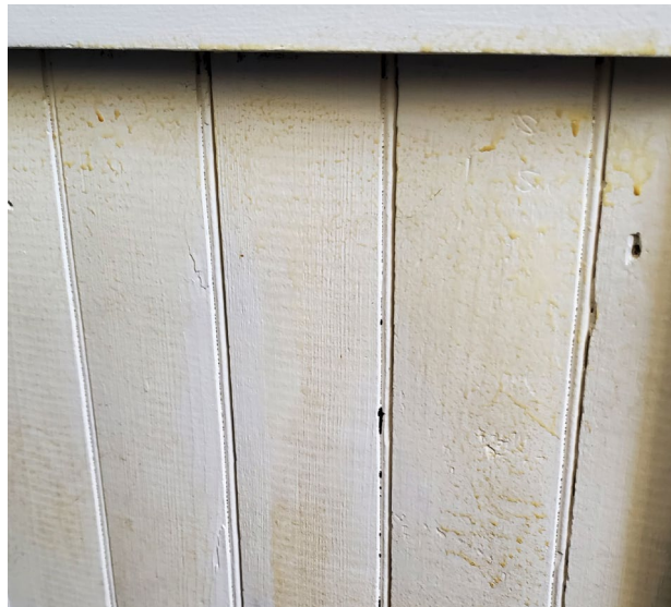
Fig. 9: Intumescent paint applied to wood wainscoting in the 1848 building. The application is not uniform.
