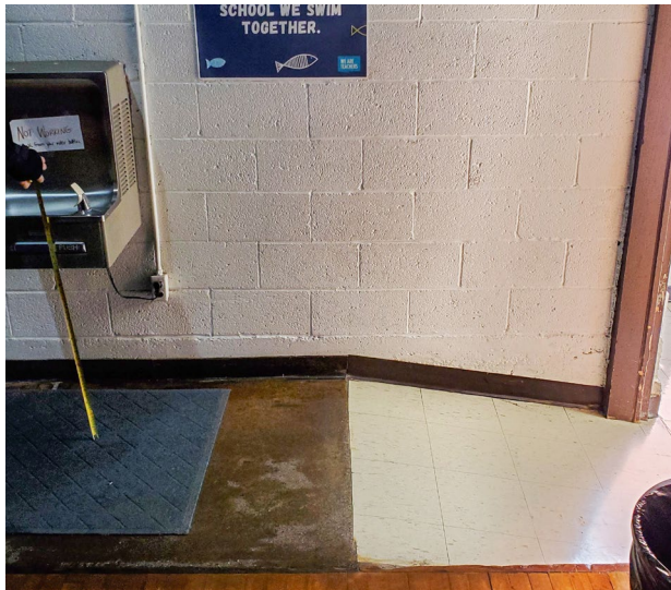
Fig. 10: A non-compliant ramp that is steeper than allowed by ADA for an accessible route. A drinking fountain projects out greater than 4" into the accessible route, which is also not allowed by ADA.
