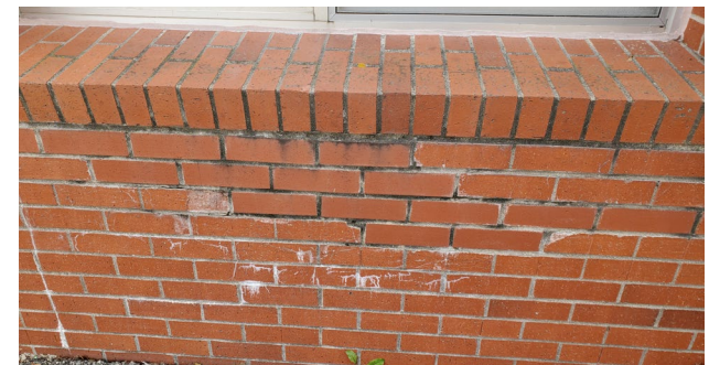
Fig. 11: Water intrusion into the 1973 brick window sill, resulting in mold, mildew, efflorescence, and deterioration of the brick and mortar.
