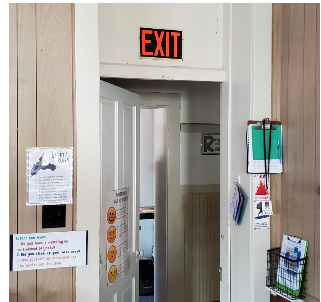
Fig. 6: No doors or windows from classrooms to corridor spaces are fire-rated. Rated doors are required in educational buildings that do not have an automatic sprinkler system installed.
